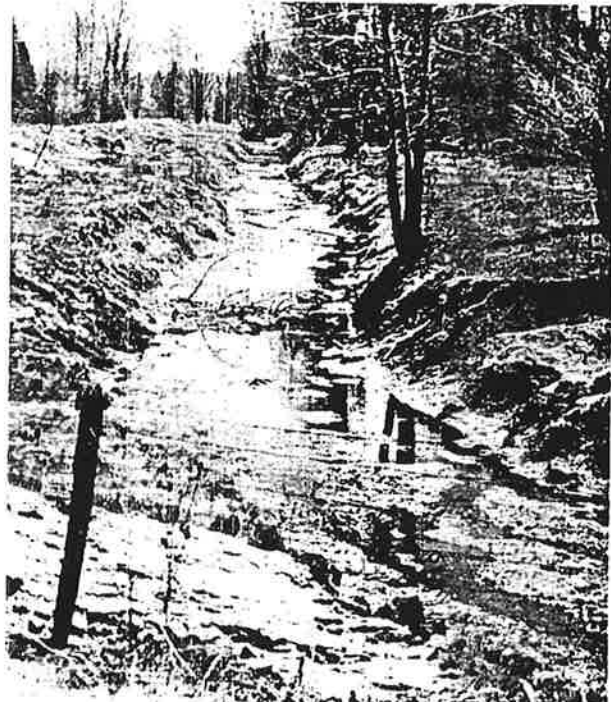
Inlet erosion and improperly leveled spoil bank.
