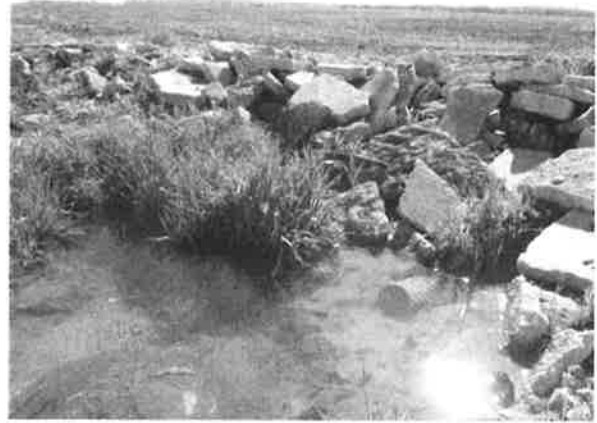
Figure B2–3. Example of an insufficient outlet.
