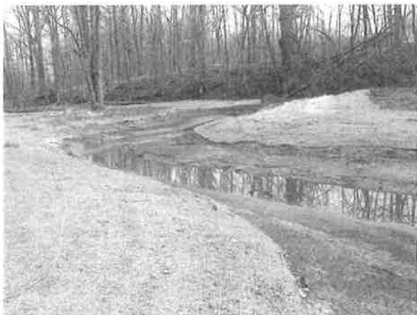
Figure B7-4. Rolled erosion control product installed on the banks of a drain.
