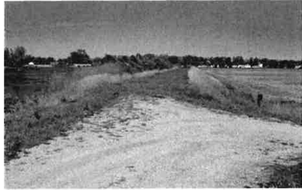
Figure B10-29. A dyke used to keep water out of the adjacent low-lying land.
