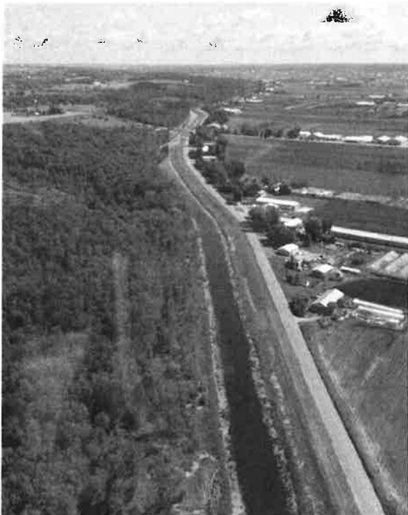
Figure B10-28. An aerial view of a dyke constructed along the full length of farmland that it is protecting from flooding.
