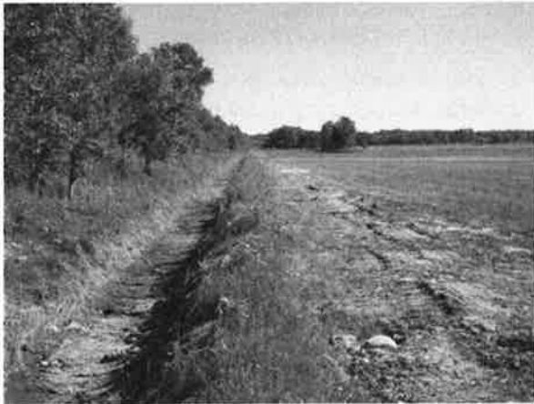
Figure B10–30. Excavated material spread to the right of the drain on farmland.
