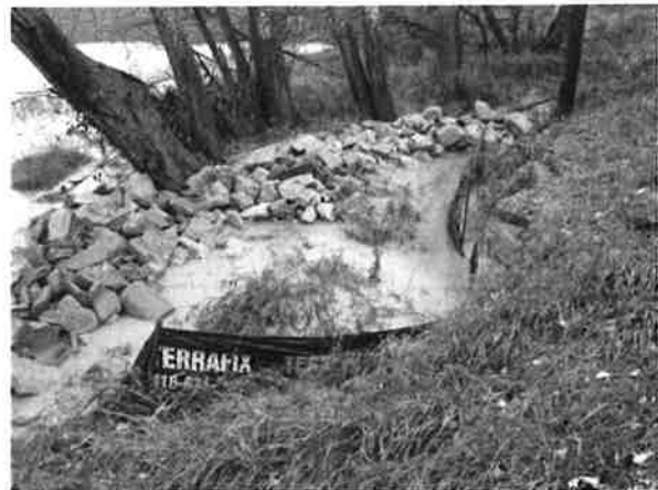
Figure B6–1. Turbid water entering a drain (due to erosion).
