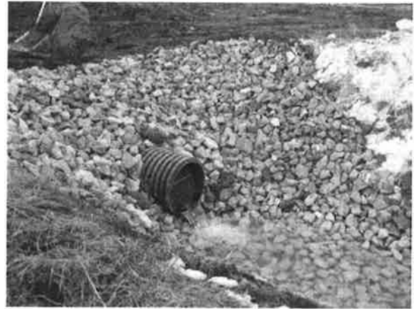
Figure B10-15. A drainage outlet.
