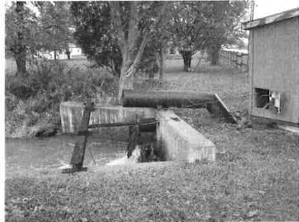
Figure B10–26. A pumping station.
