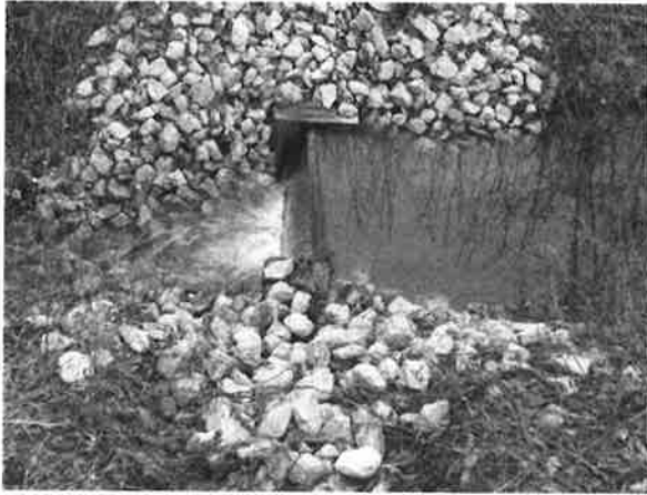
Figure B8-3. A water control structure.
