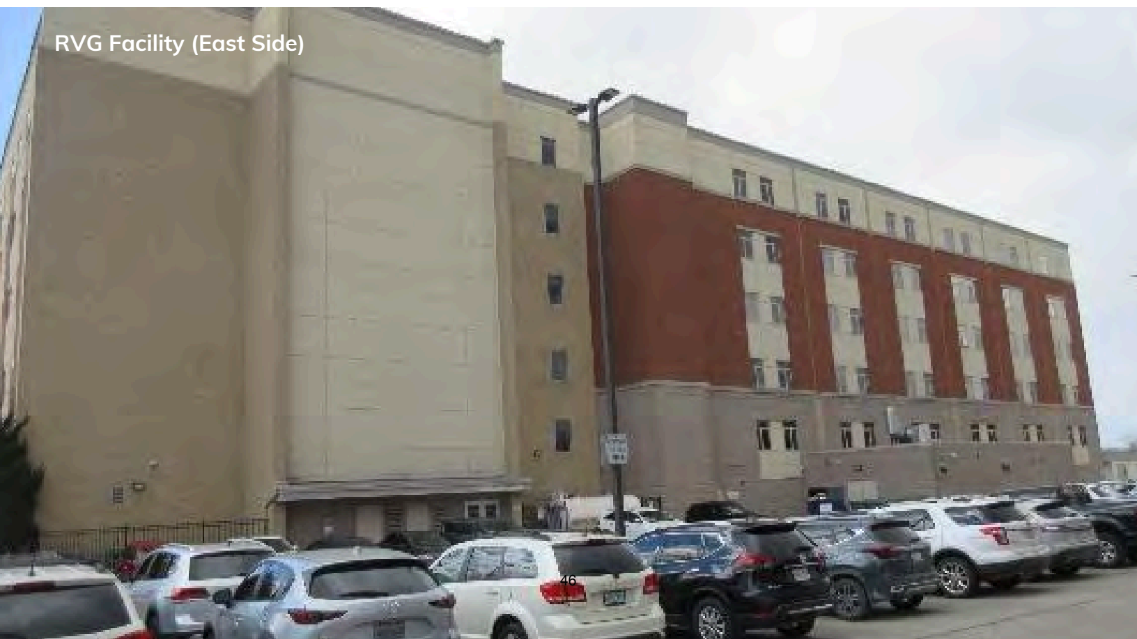
RVG Roof with pooling water
