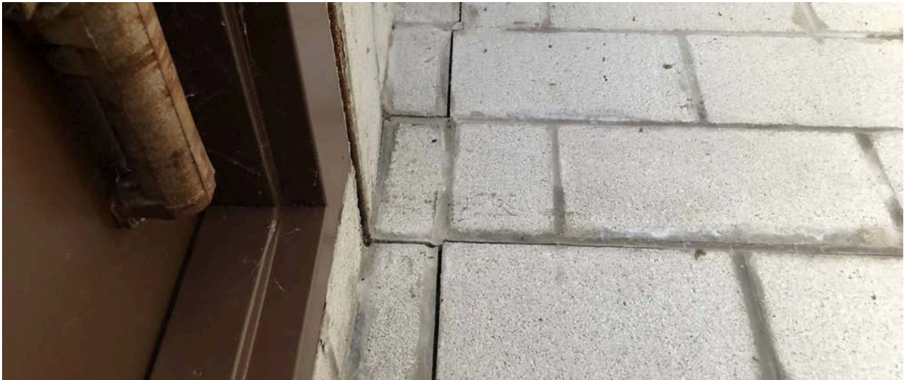
Cracking concrete block wall within maintenance garage
