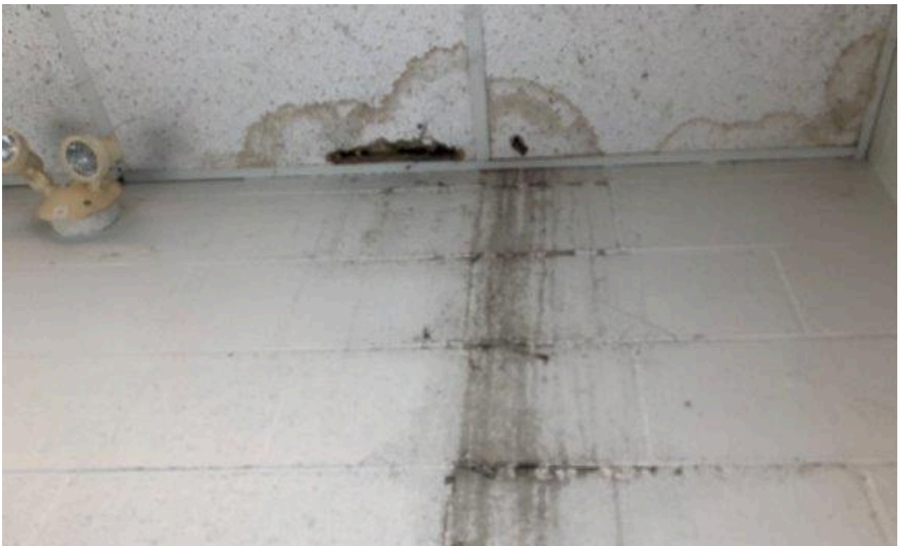
Water leak through a ceiling-tile
