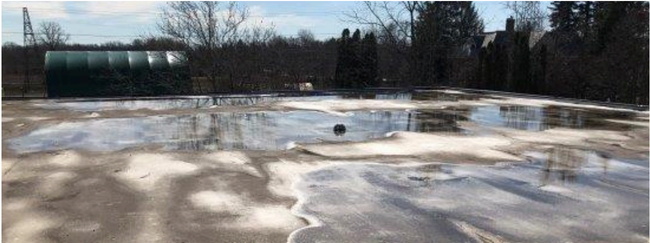
Pooling water on an aged-roof
