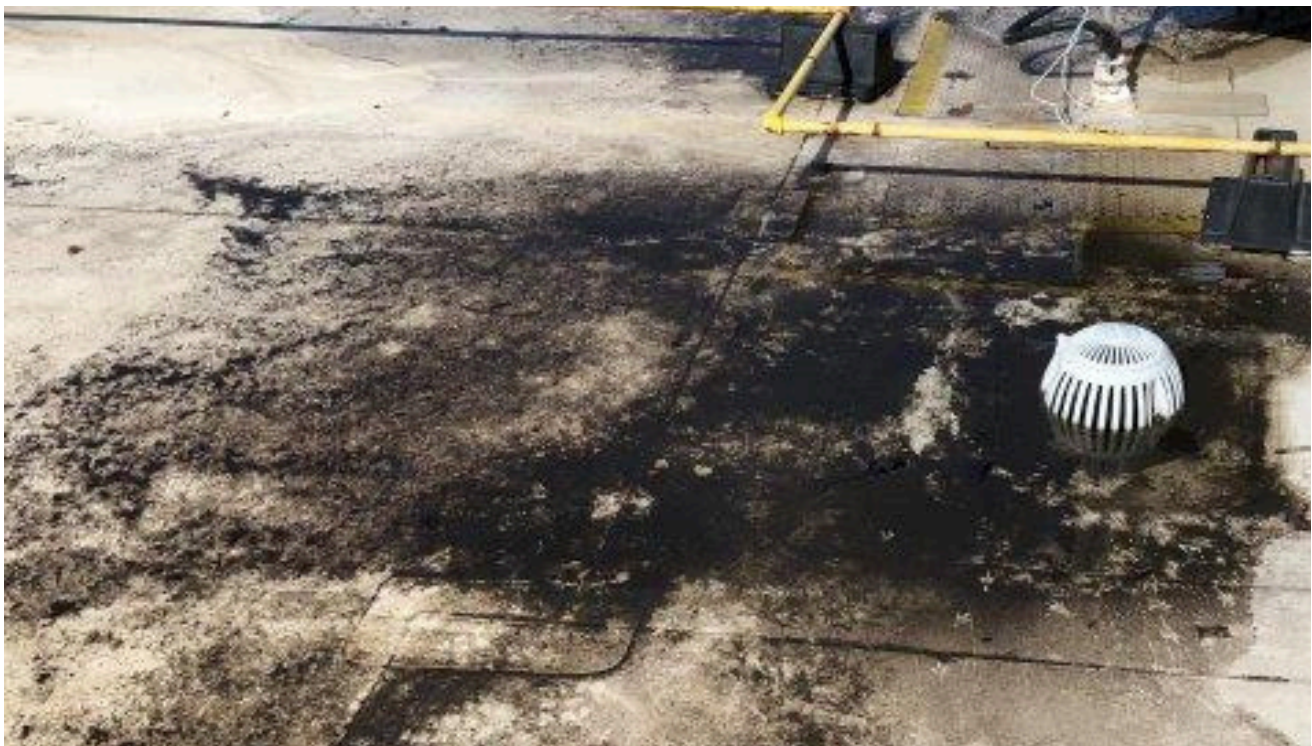
Clogged roof drain and pooling water
