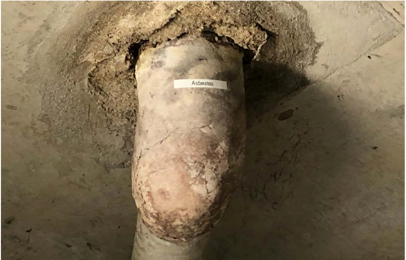
Asbestos-containing parging cement on piping
