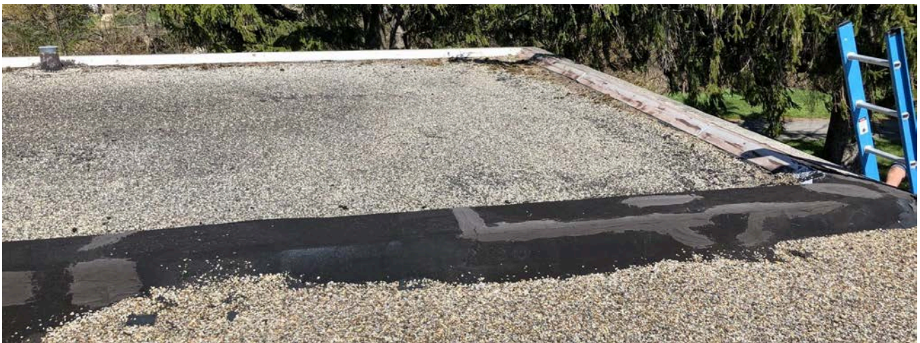
Roof of maintenance garage requiring replacement
